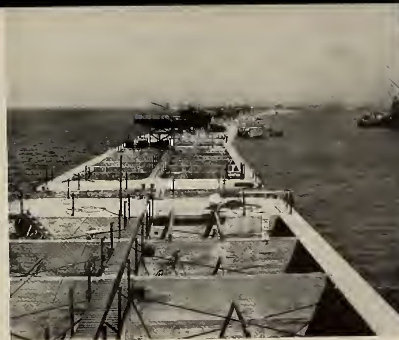
4. The caissons were placed in a continuous row. They were built in six different sizes for different depths of water. The biggest displaced 6,044 tons, the smallest 1,672 tons. Note the sea-cocks used to let in the water to sink them in position. Dredge ships also pumped sand into the compartments. For protection against enemy air attack anti-aircraft guns were mounted on the biggest caissons and barrage balloons floated overhead. Quarters for the A-A gun crews were built on the caissons.
